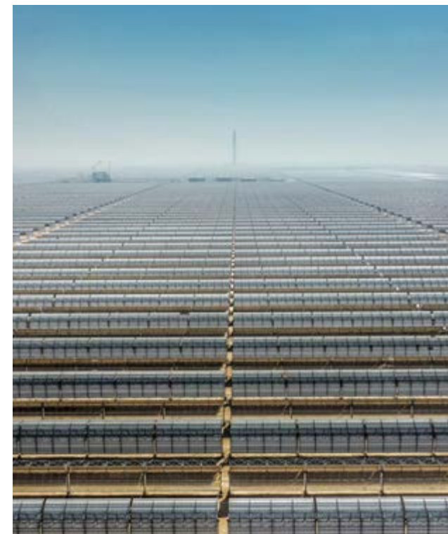
► Abengoa has completed the construction of a parabolic trough solar field for the largest solar complex in the world, in Dubai.
