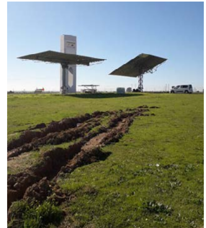
► Detail of heliostats at the Pontones test platform.
