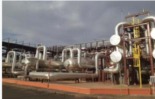
► Kaxu Solar One solar steam generator.
