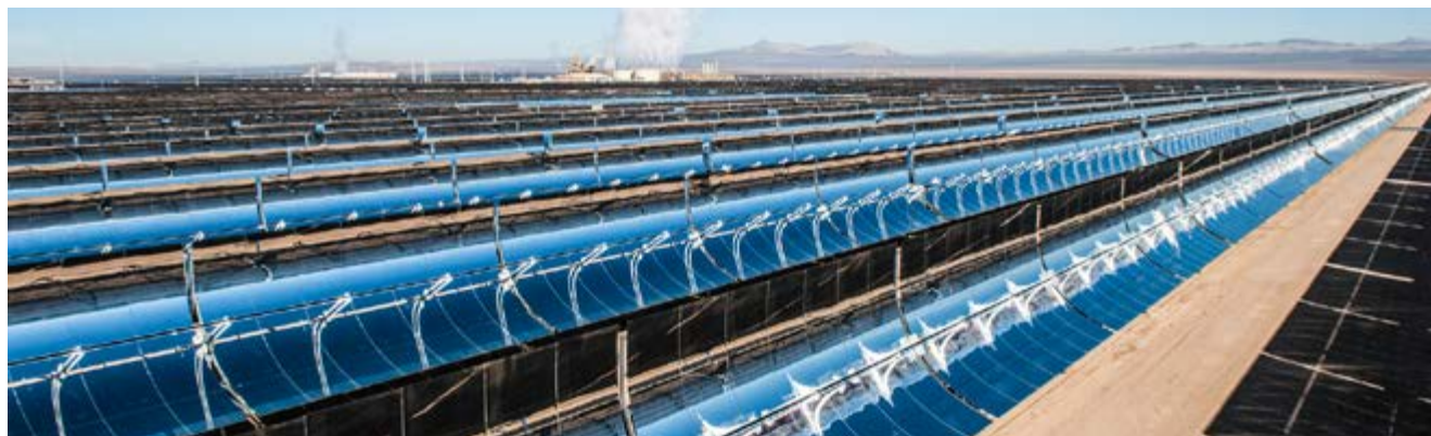
▶ Abengoa is engaged in the Scarabeus project on supercritical CO 2 to increase the efficiency of solar thermal plants.
