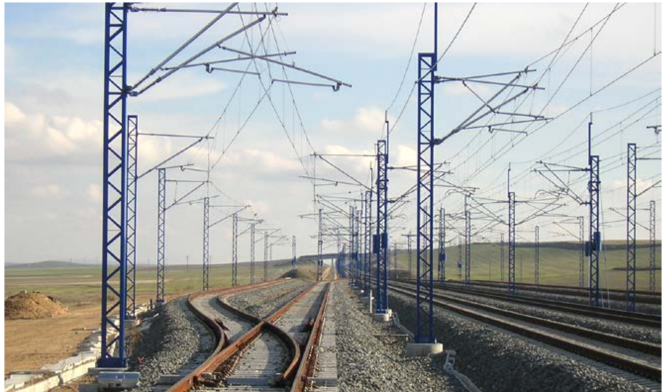
► The Alis innovation project provides safety and efficiency to railway systems.
