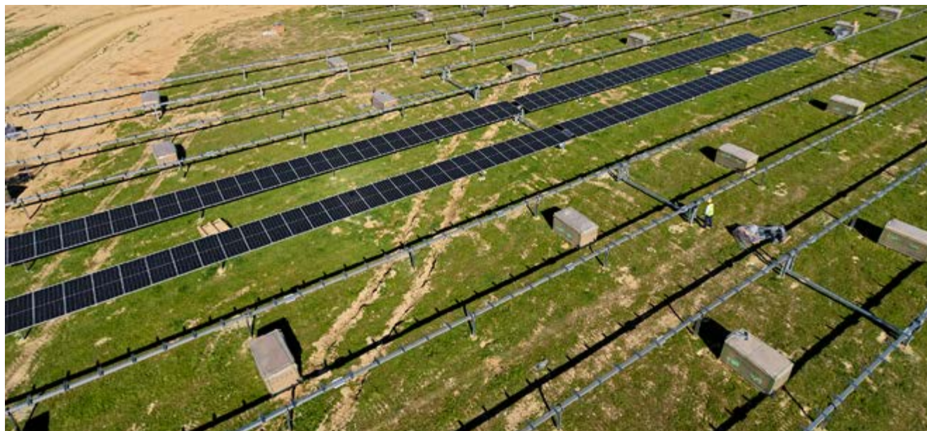
► Abengoa and FCC are building the largest photovoltaic project in Europe in Cáceres (Spain).
