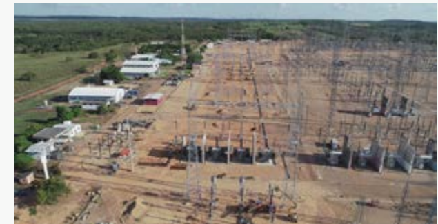
► The company has been awarded the civil works and assembly of the 500 kV Miracema substation.
