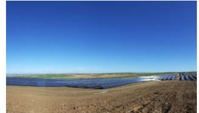
► Abengoa is developing the construction engineering for a photovoltaic plant in Barciencia (Toledo).
