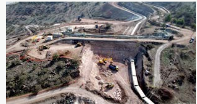
► Civil works on roads, electric fences, laying and replacement of transportation pipelines for Codelco in the Andina division.
