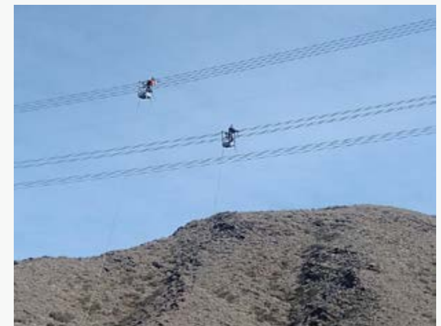
► Placing spacers on 500 kV line laying, in the province of San Juan.
