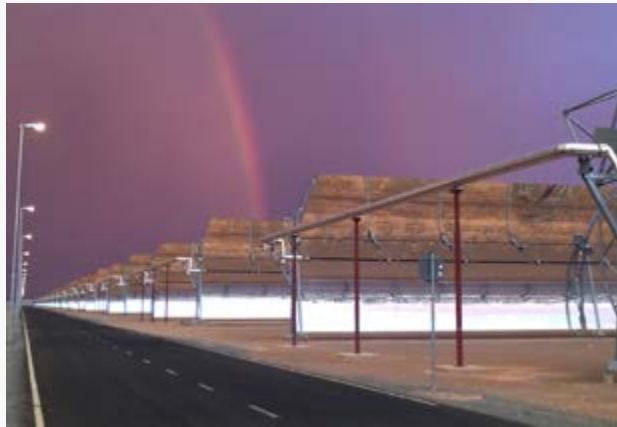
► Partial view of the Xina Solar One solar field with a large-opening parabolic trough collector.
