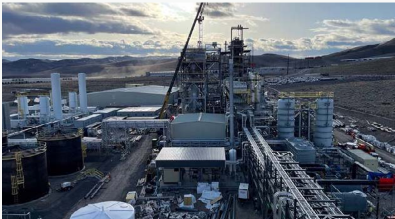
► Abengoa continued the construction of the Sierra Biofuels plant for Fulcrum during 2020.
