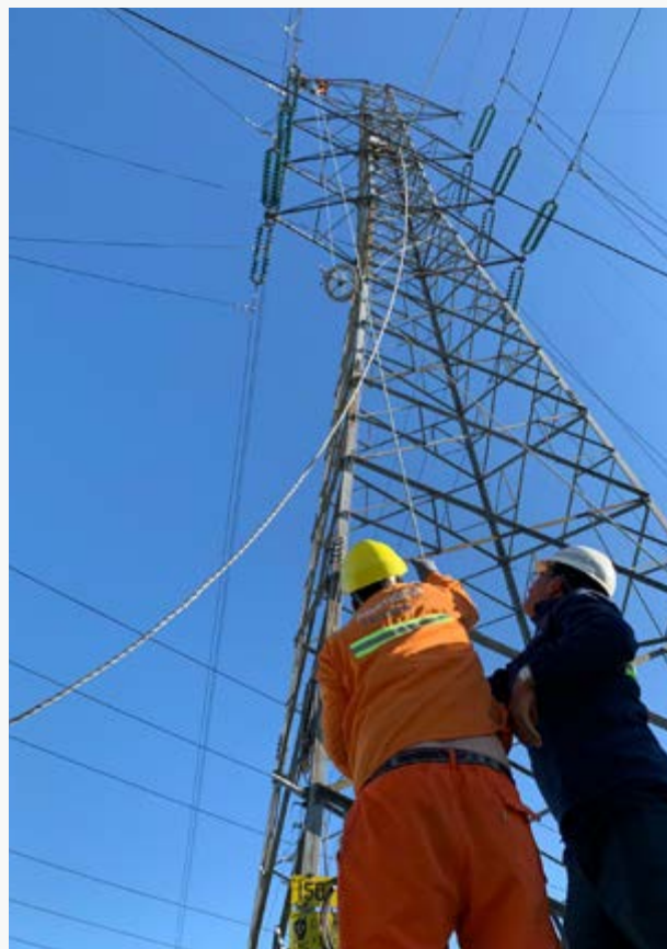
► Last year, the company completed the laying of OPGW (Optical Ground Wire) fibre optic cable on a 150 kV line.
