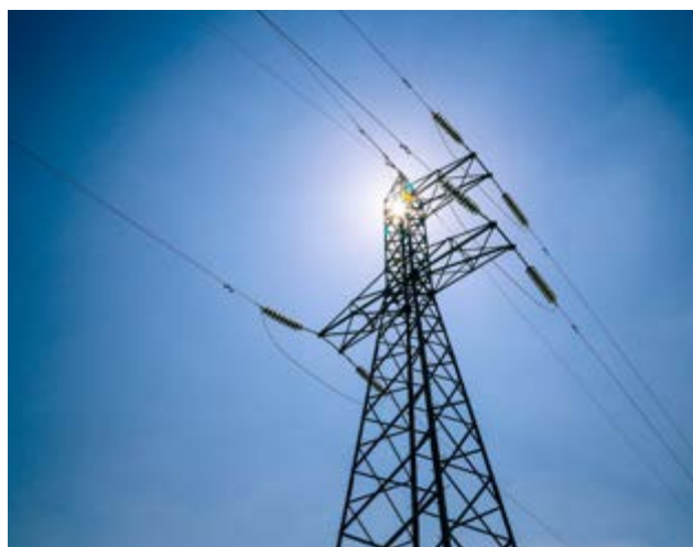
► Abengoa is an international leader in transmission and distribution with more than 27,000 km of lines and more than 330 substations built in the last 15 years.
