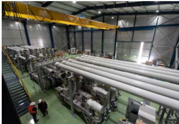
► The 345 kV Altiplano switching station, with AIS and GIS technology and specific designs due to its location at 4,000 meters above sea level, became operational in 2020.
