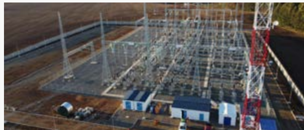
► During the last year, Abengoa completed the construction of the 220 kV Malleco substation.
