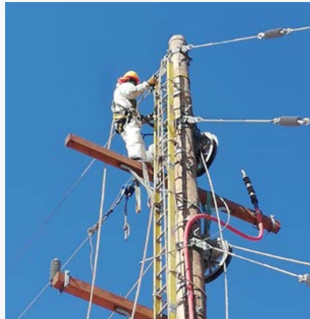
► Work on the distribution line of the Minas Justa de Marcobre mining project.
