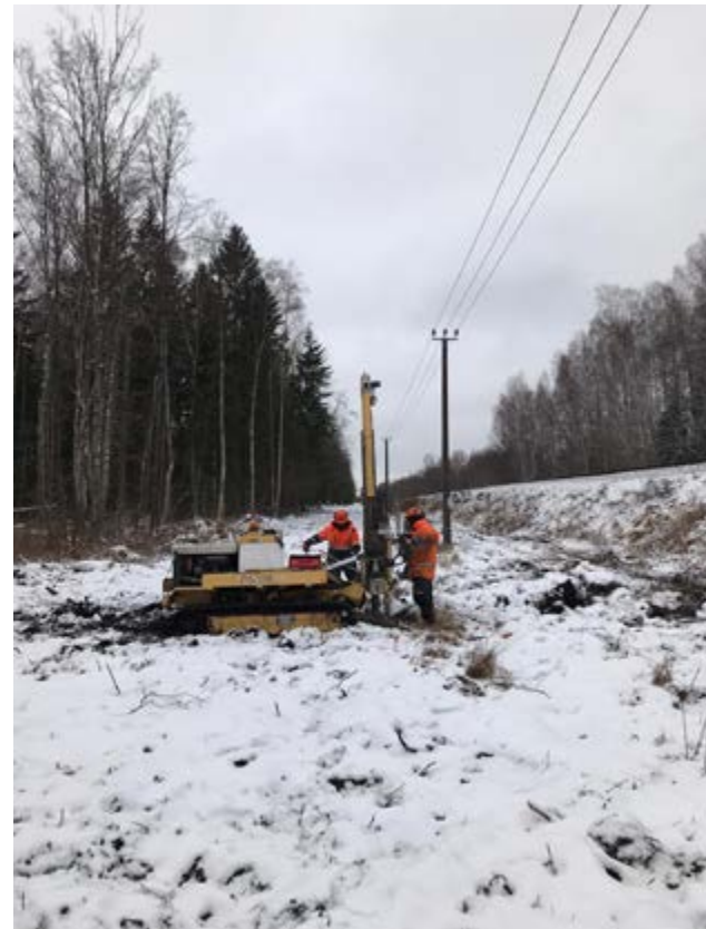
► Abengoa is working on a railway electrification project in Lithuania to connect the country from east to west.
