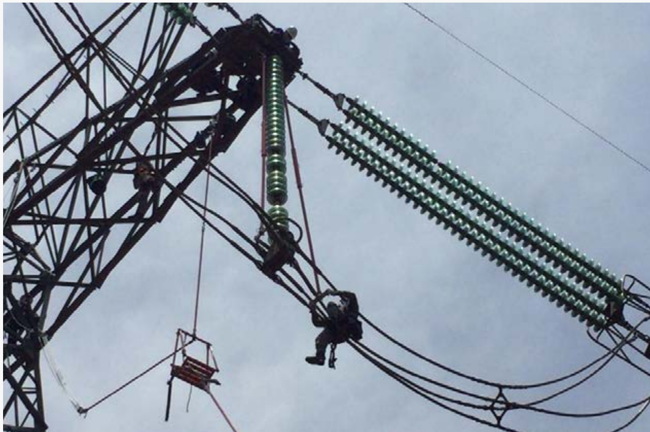
► Abengoa has created a live line maintenance area (energized).
