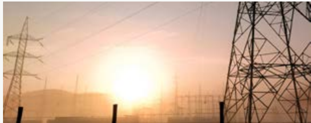
► Abengoa's 220 kV line constructed for Arauco in its MAPA project.
